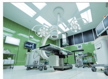
Hospital Emergency Power
