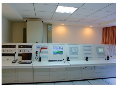
Auto Control System
