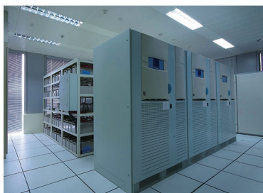
Electric Power System (EPS)
