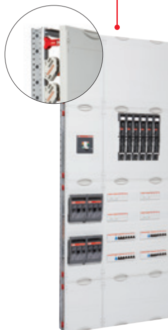
Assembly with WR mounting frame* Internal configuration as sub-distribution board with CombiLine modules on WR mounting frame
