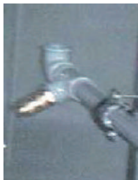
Compressed air installation
