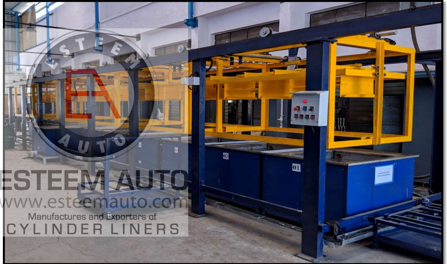
10 Tank automated phosphating plant
