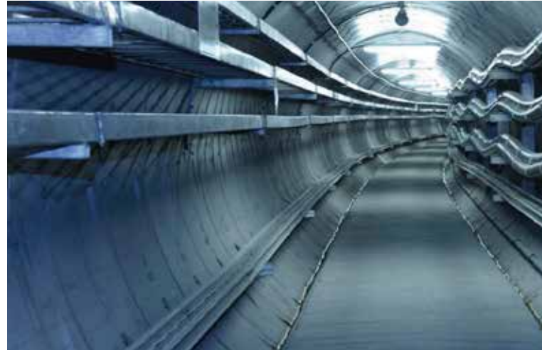
SPPG Cable Tunnel, Singapore
