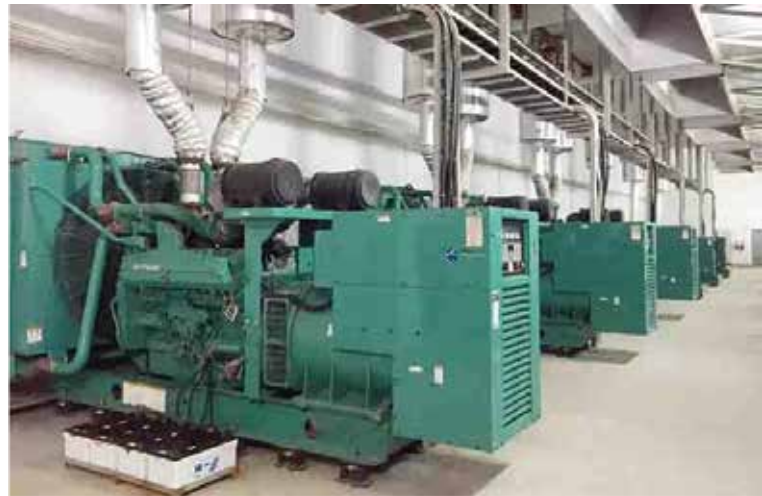
PSA AA Generator Containers & Transformers, Singapore
