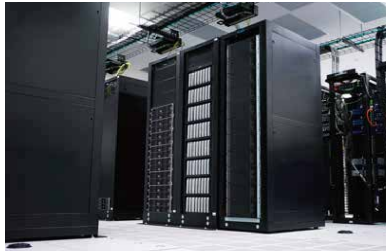
Shanghai Bank Data Centre
