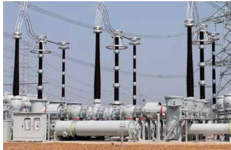
230kV Substation, Southern Aluminum Smelter, Iran
