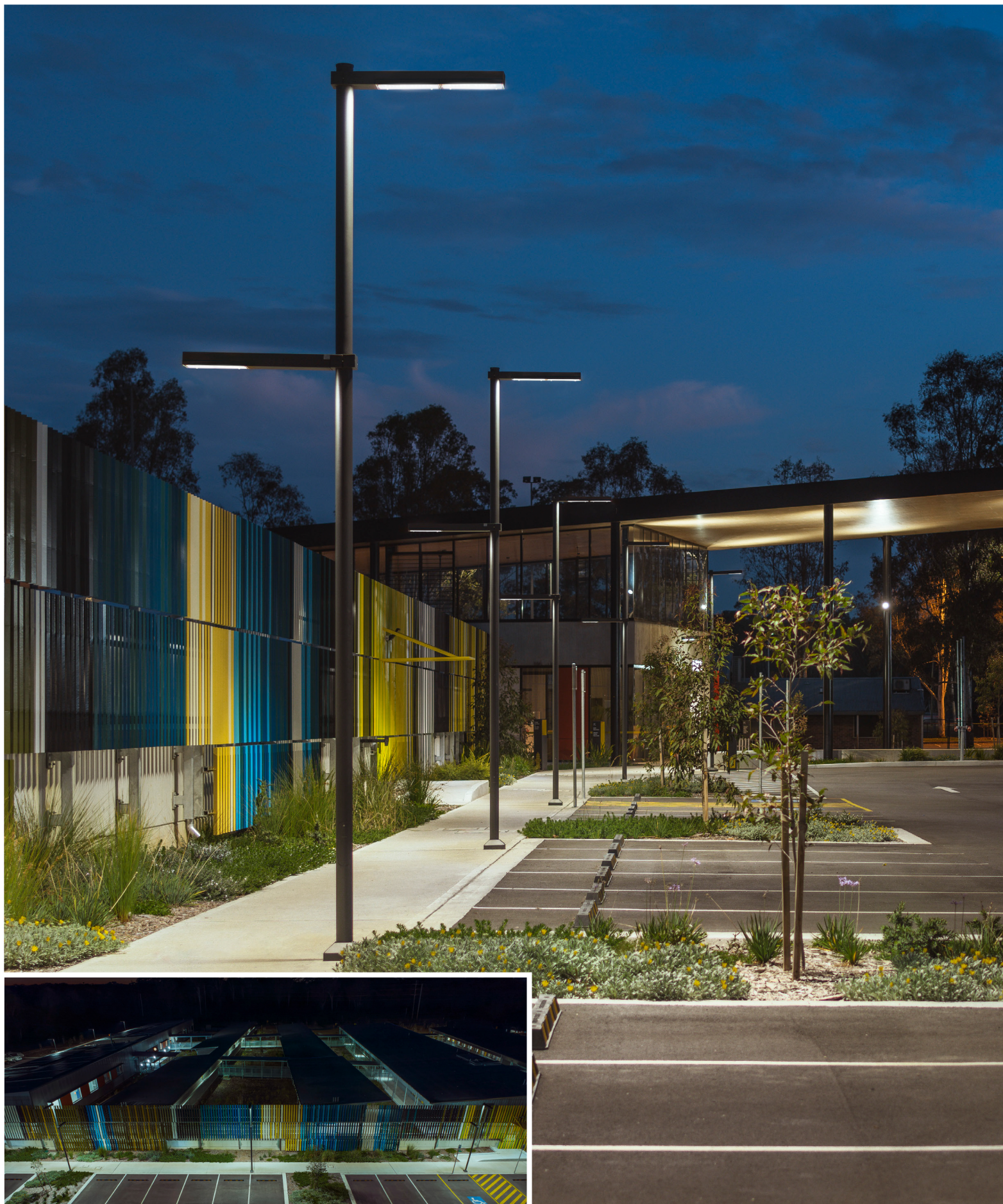
Light Linear Pt Street & Area Luminaire | Bankstown Animal Rehoming Centre NSW, Australia
