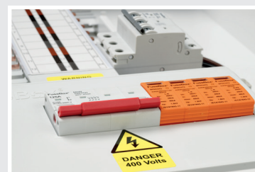
SPD mounted beside main switch
