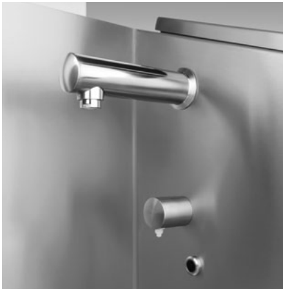
Detail: Outlet tap and soap dispenser
