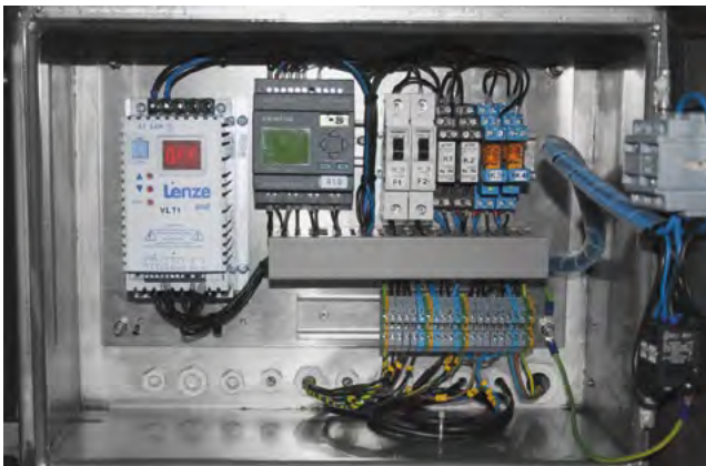
High-quality control cabinet components
