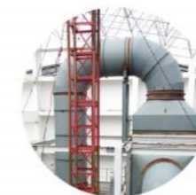
Energy Saving & Emission Reduction (Low-temperature Waste Heat)
