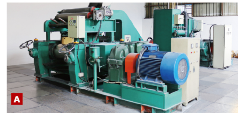
A Rubber material mixing production line B Automatic weighing feeding system C Small material weighing system
