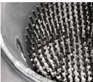
ECOTHERM high capacity water heaters after 12 months in operation: almost no lime scale.
