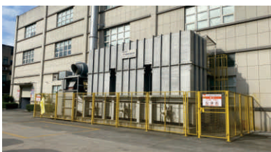
RTO Regenerative Oxidation Furnace
