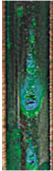
Internal Corrosion – Copper
