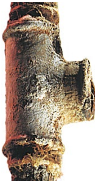
External Corrosion – Galvanised Steel
