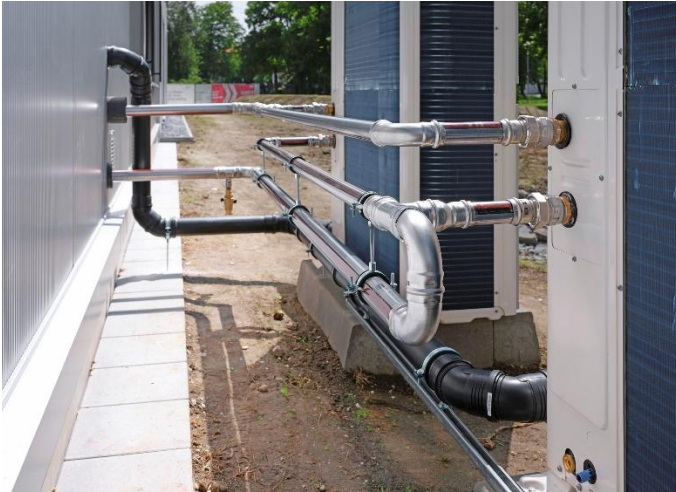
Image 3 (PR_ISH_Connection_HeatPump_EN_2025-03): Monobloc heat pumps installed outdoors can be easily connected to the hydraulic station in the house thanks to the appropriate connection sets from Viega's "Temponox" stainless steel press connector system. (Photo: Viega)
