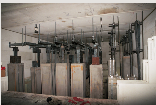
Fire inspection before.
