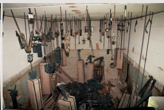
Fire inspection after.
