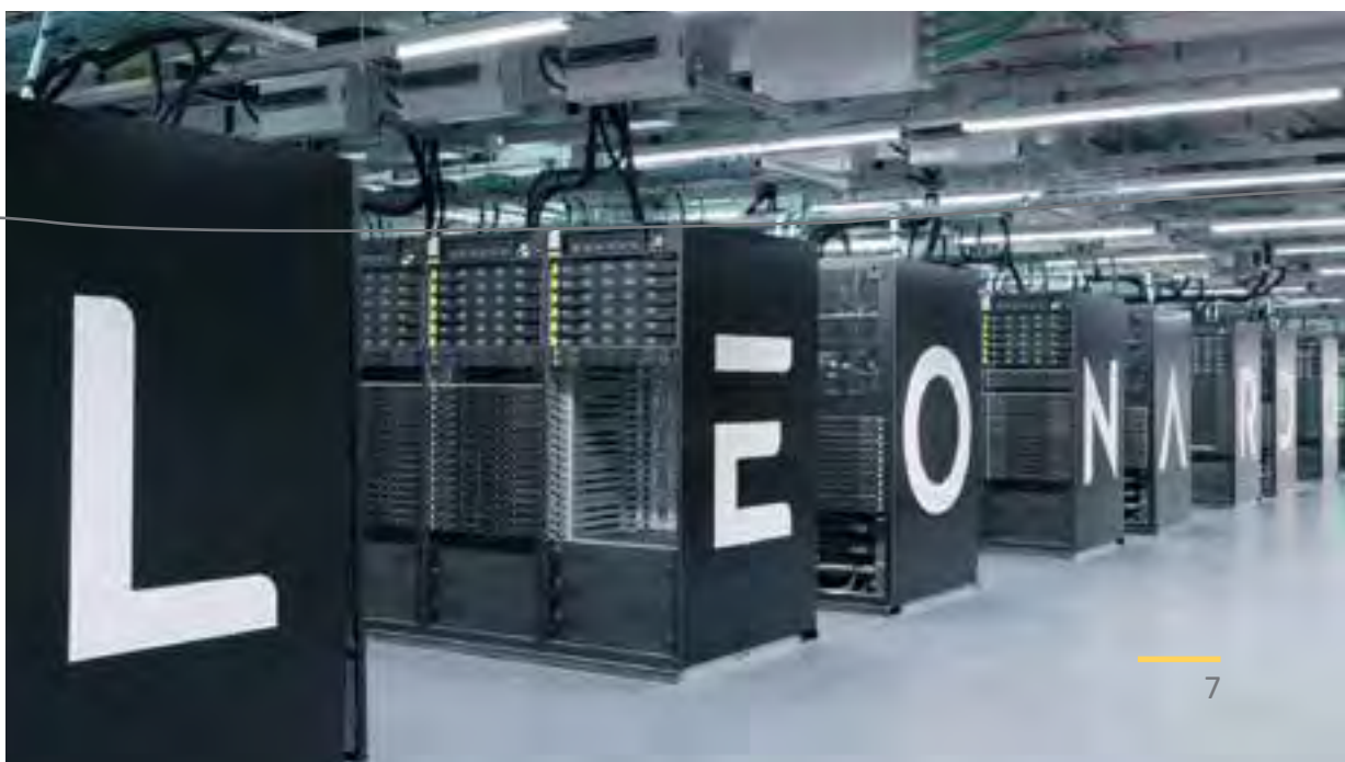
LEONARDO - BOLOGNA ITALY - 2022 Heating/cooling system
