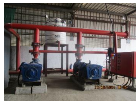
Fire hydrant system pumps
