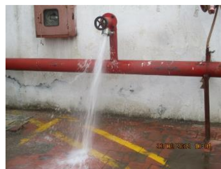
Fire hydrant point tested
