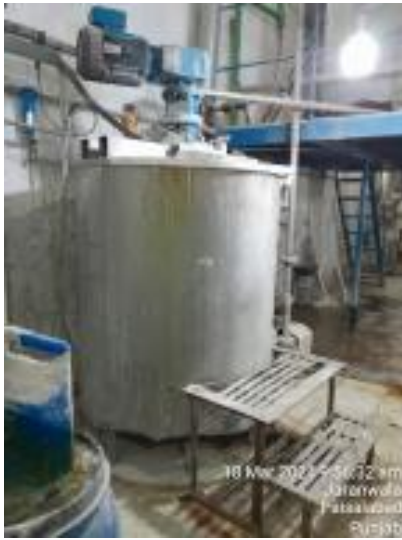
Non-conformance - Chemical Drum without labelling.jpeg
