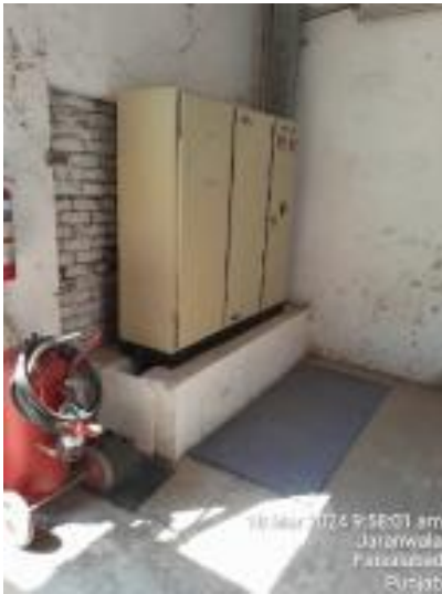
Non-conformance - Electrical DB without danger sign 2.jpeg
