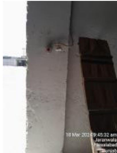
Non-conformance - Fire Alarm not identified.jpeg
