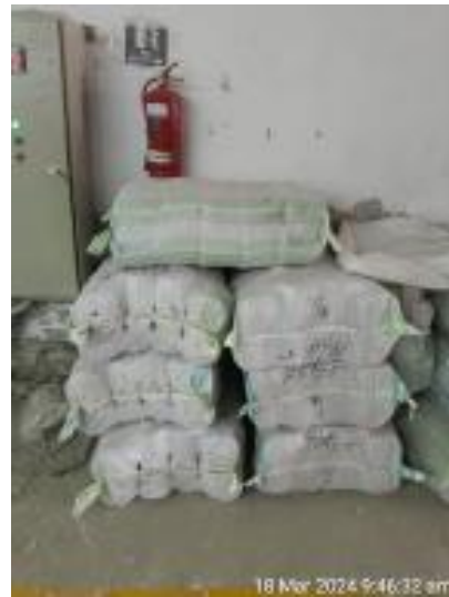
Non-conformance - Fire Extinguisher Blocked.jpeg
