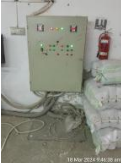
Non-conformance - Electrical DB without danger sign 1.jpeg
